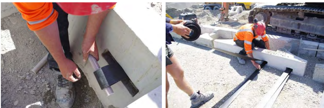
GFRP Paraweb pin installation – form loop in Paraweb, thread through connector, install pin and pull back to lock into place. Ensure pin has a tight fit into connector – may need a hammer tap to seat properly.
