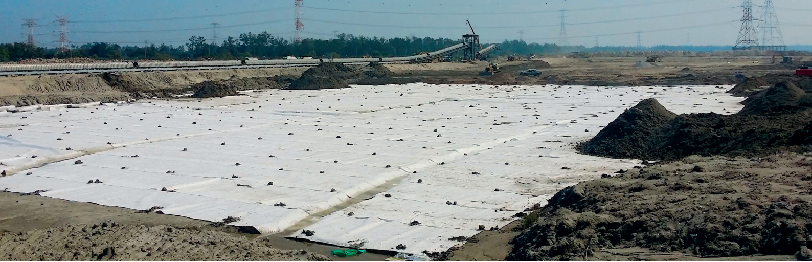
Fig.1: Installation of Combigrid® with trench for collector pipe and regulating sand backfill
