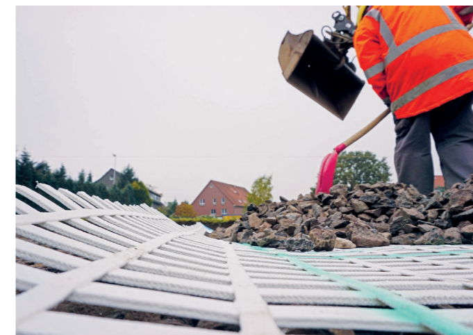
Figure 4: Field trial with Secugrid® HS to determine the installation damage ( RF_{CR} ) reduction factor
