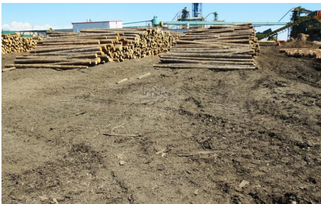
Photos showing log yard before (top and middle) and after (bottom) installation of Neology Geocell
