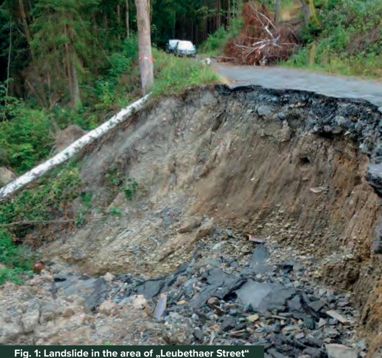
Fig. 1: Landslide in the area of „Leubethaer Street“
