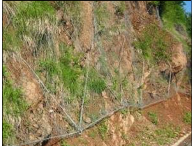
Steel Rope used to reinforce the mesh and secure the net at the toe of the slope
