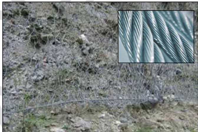
Steel rope used to fix the net at the base of the slope
