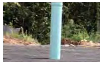
Fig. 16 Installed maintenance port
